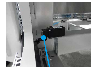
Belt cleaning unit position sensor
