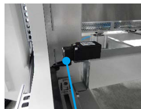
Belt cleaning unit position sensor
